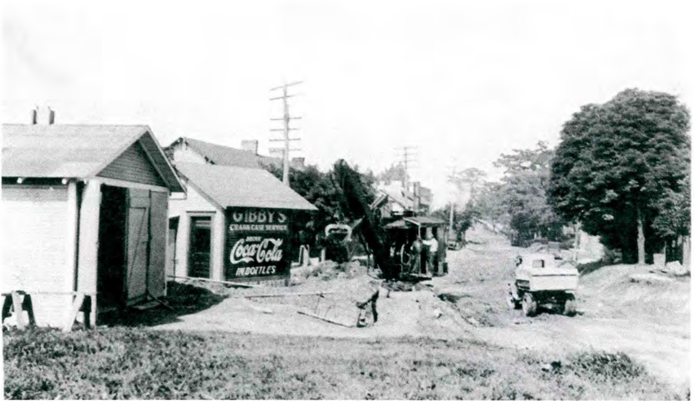
Steam shovel in operation at the corner of Rt. 18 South and Rt. 22 East Looking towards Rt. 22W (upper left) and Rt. 18N (upper right)
