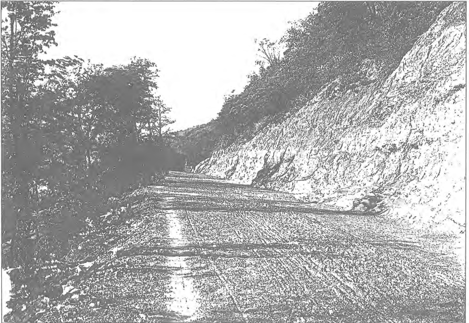
Preparation for the street car lines to connect the future WV Rt. 2 to Steubenville, Ohio.
