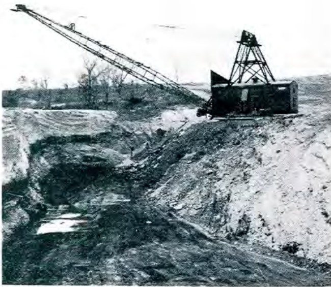
The second stripping unit is this electric walking dragline, shown here operating from the spoil bank side of the pit. Equipped with a 165-ft boom and a 12-cu-yd bucket, this unit has been in use since 1944.
