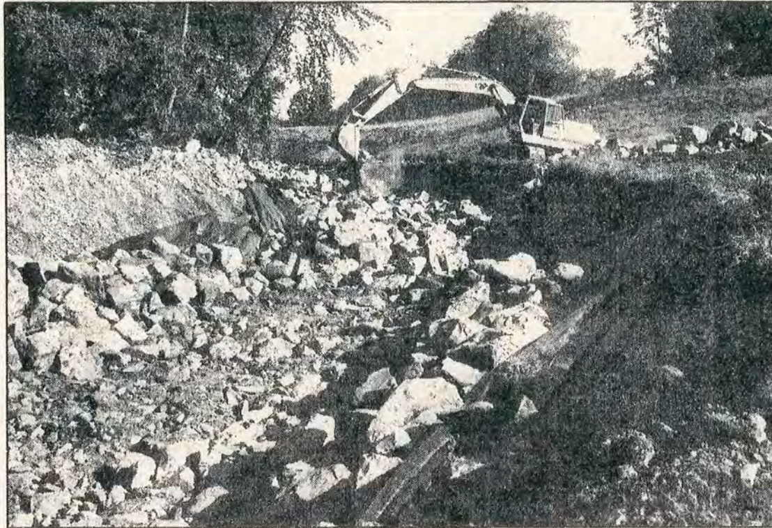
A BACKHOE OPERATOR works on a rock channel designed to control erosion in the Cedar Grove area of Cross Creek Township.
