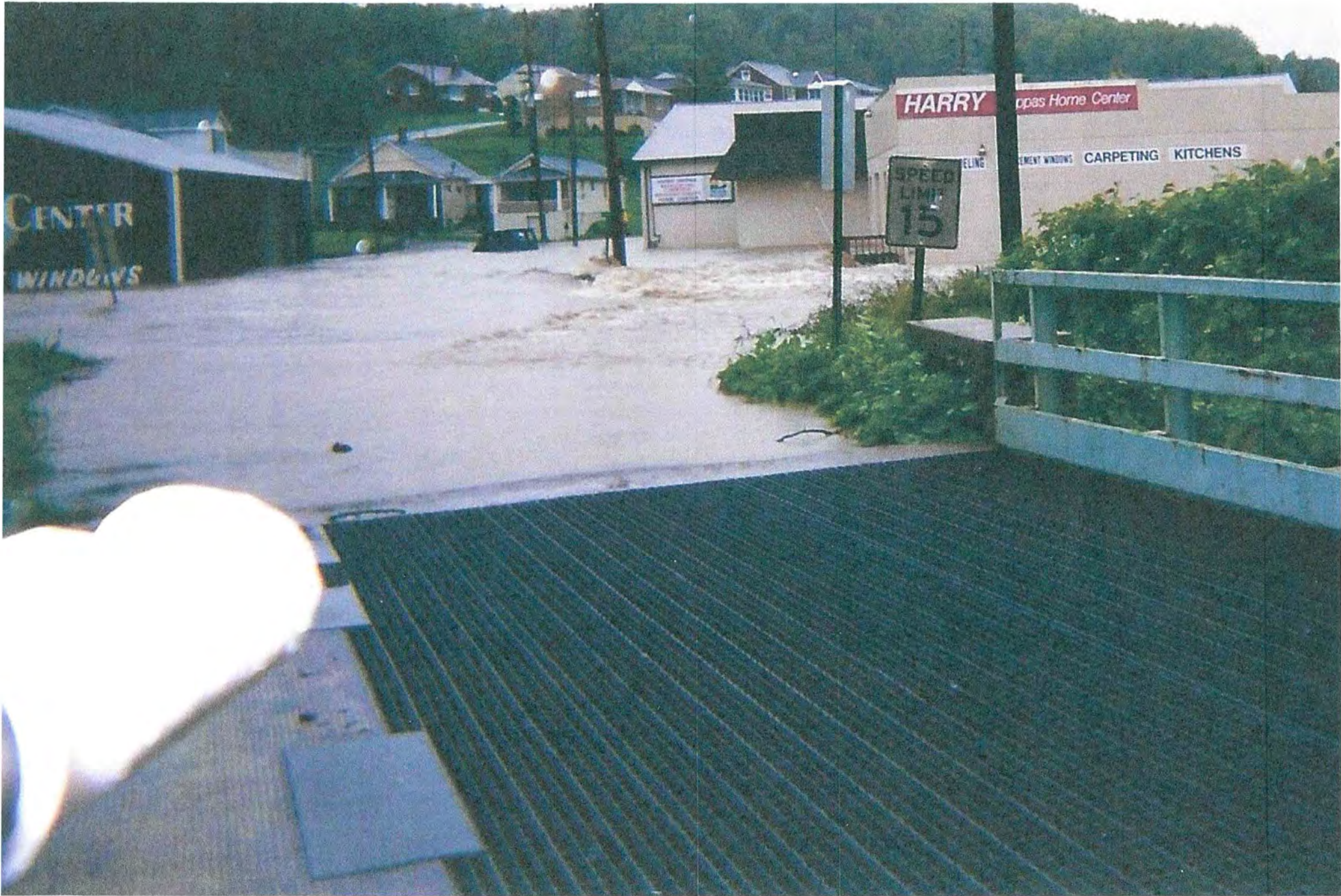
West Pittsburgh Street bridge near Harry Pappas Home Center Burgettstown, PA -September 17, 2004
