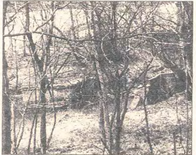
ONLY THE PIERS remain where the railroad once crossed near Pattersons Mills. A flood in 1912 swelled through Cross Creek Valley destroying most of the remaining railroad .
