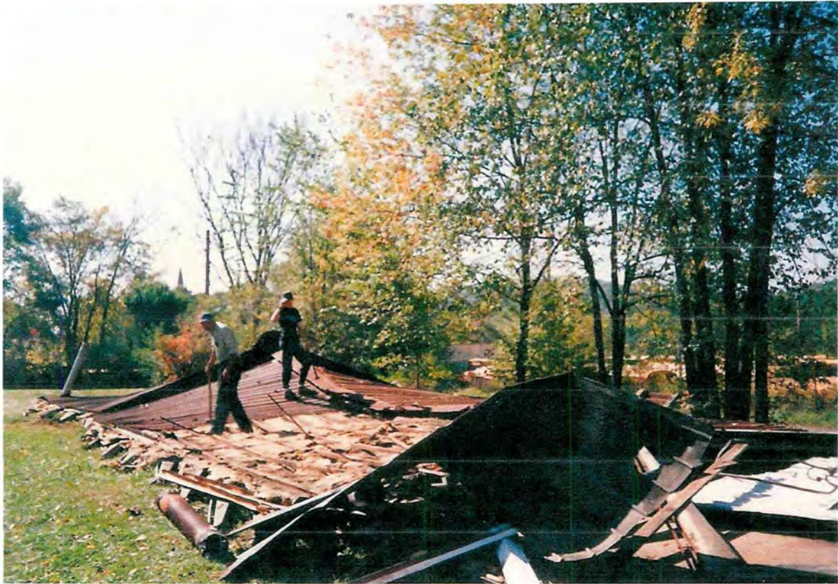
Former Metal Maintenance Shed for the Old Burgettstown High School being torn down. Located behind the Burgettstown Community Library-1995
